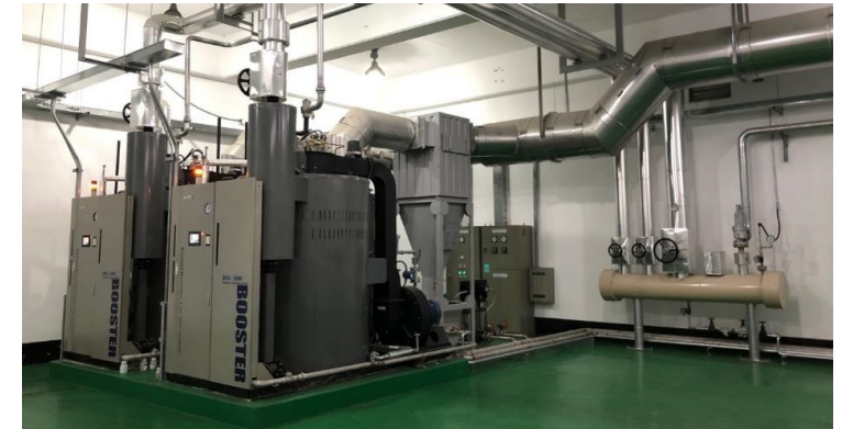
Low NOx Kerosene Boiler at the Logistics Center in Busan
